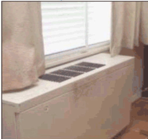
Mold growing on the surface of a unit ventilator.
