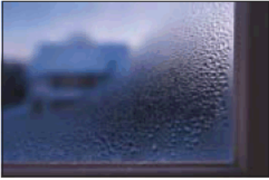
Condensation on the inside of a windowpane.
