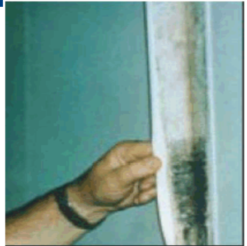
Mold growing on the back side of wallpaper.
